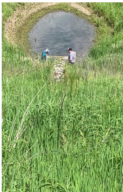
Bryan Shupe, DC, and Dallas Steele, State Technician, check the condition of the overflow outlet at the Anderson Conservation Area flood control basin.
