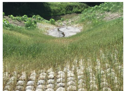
Top to bottom: Shaping the ditch; laying down FlexaMat® bricks; vegetation growing through mesh; view down chute toward river.
