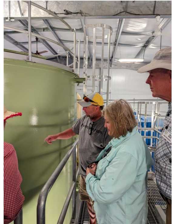
Plant Operator Todd VandeKop reviews Lyon & Sioux Rural Water treatment plant processes with CDI President Jeri Thornsberry and CDI Region 2 Director Perry Black.
